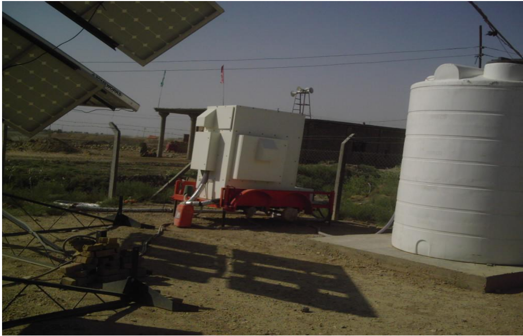
Fig. 9. Desalination unit and reservoir with solar panel
