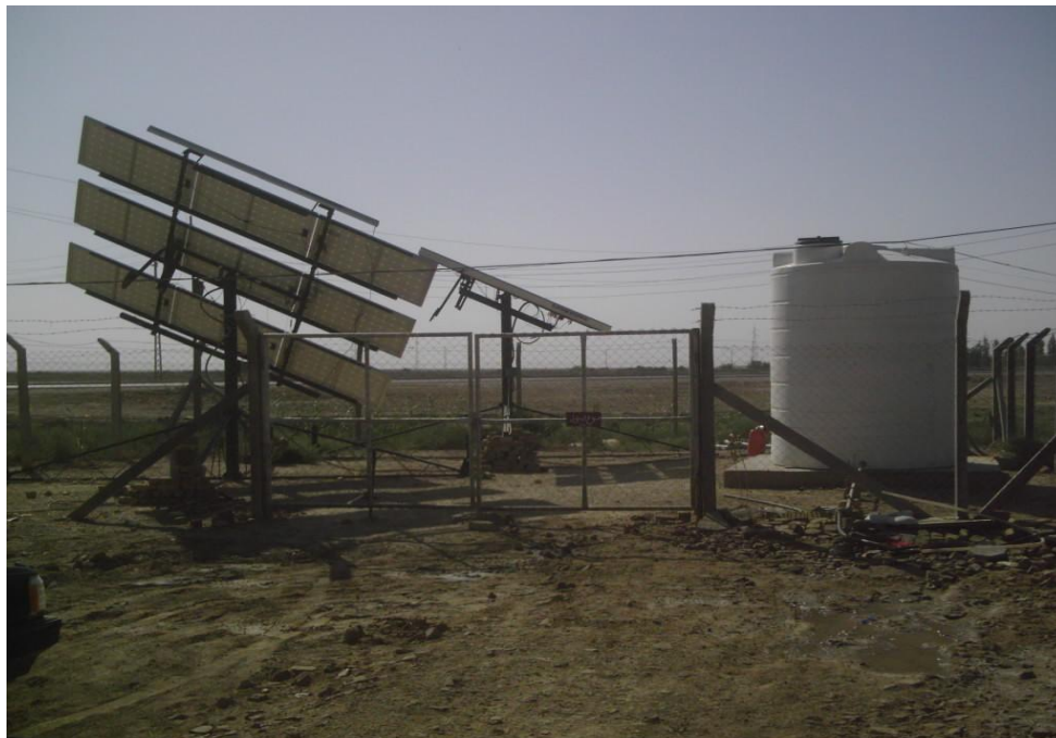
Fig. 8. Solar panels and 10000 liters water reservoir
