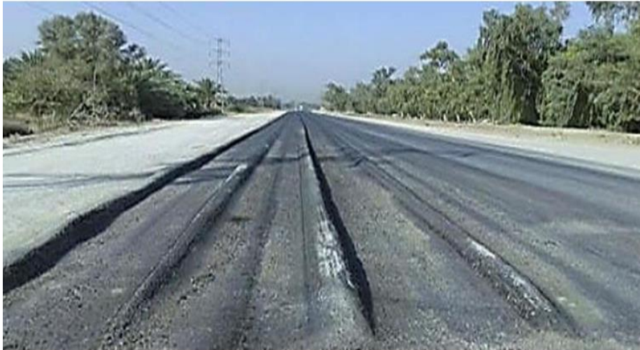
Figure 1. Rutting occurring in pavement (the road located in Iraq)
