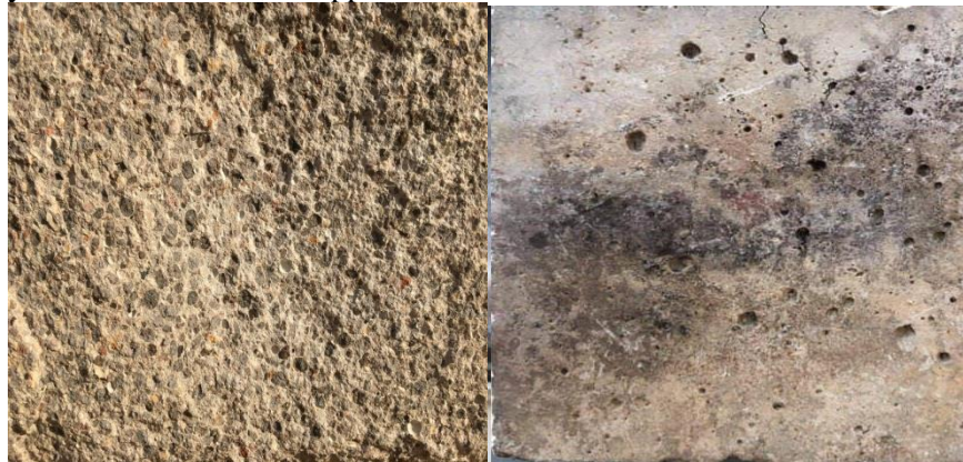
Figure 12. Speckle pattern of tested beam, A- Specimen surface enlarged image, B- Partial enlarge hairline cracks
