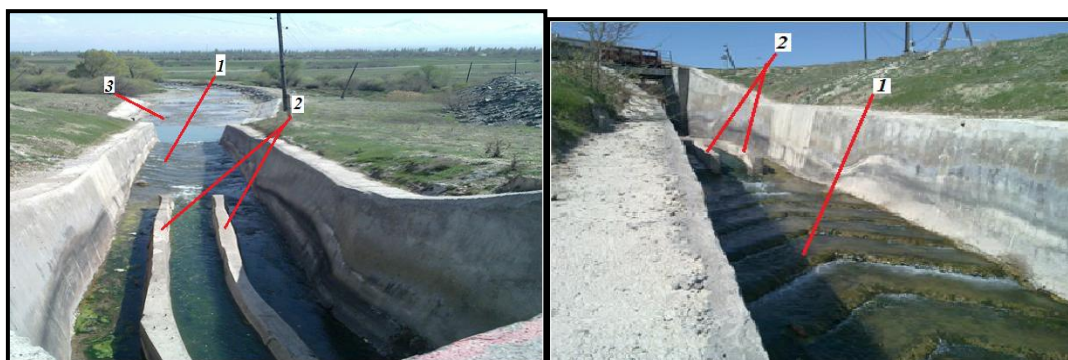
Figure 1. Spillway channel with artificial roughness in the Ters-Ashchibulak reservoir (views of the upper and lower reaches): 1 – artificial roughness; 2 – partitions; 3 – discharge channel (downstream)
