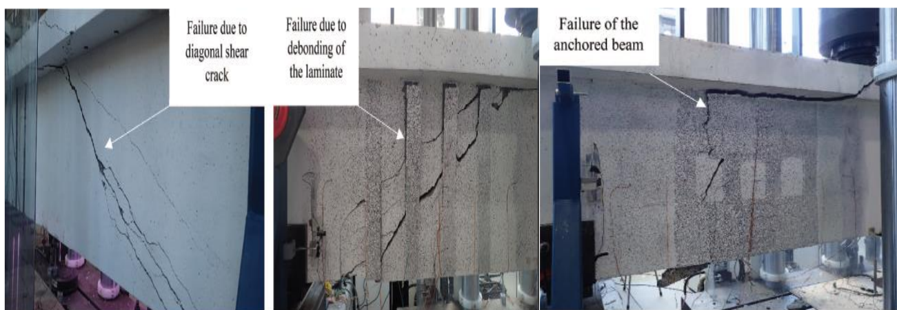
Figure 1. Summary of the failure of PSC beams strengthened by CFRP [4]
