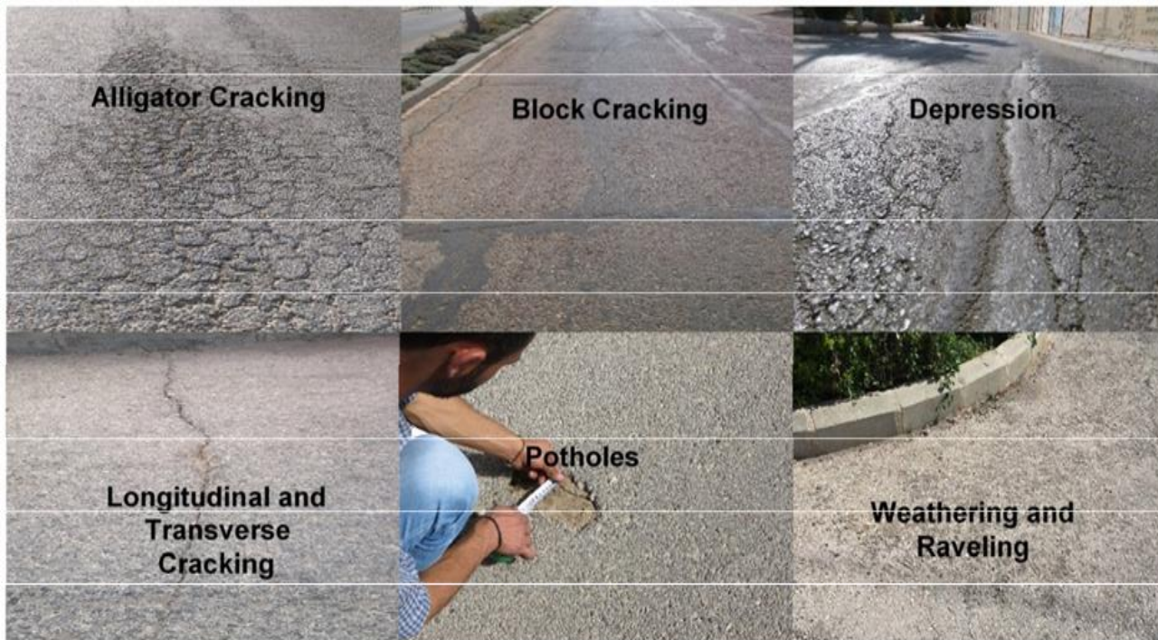
Figure 5. Types of pavement cracks during data collection
