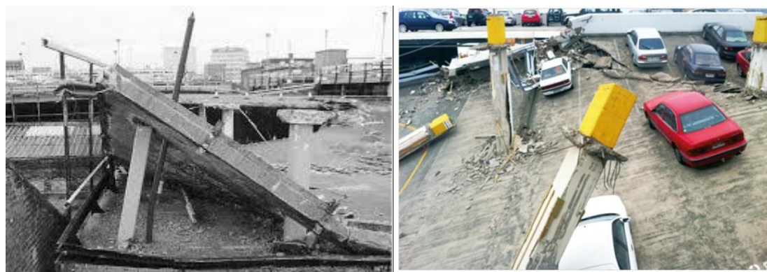
Figure 1. Punching shear failure
