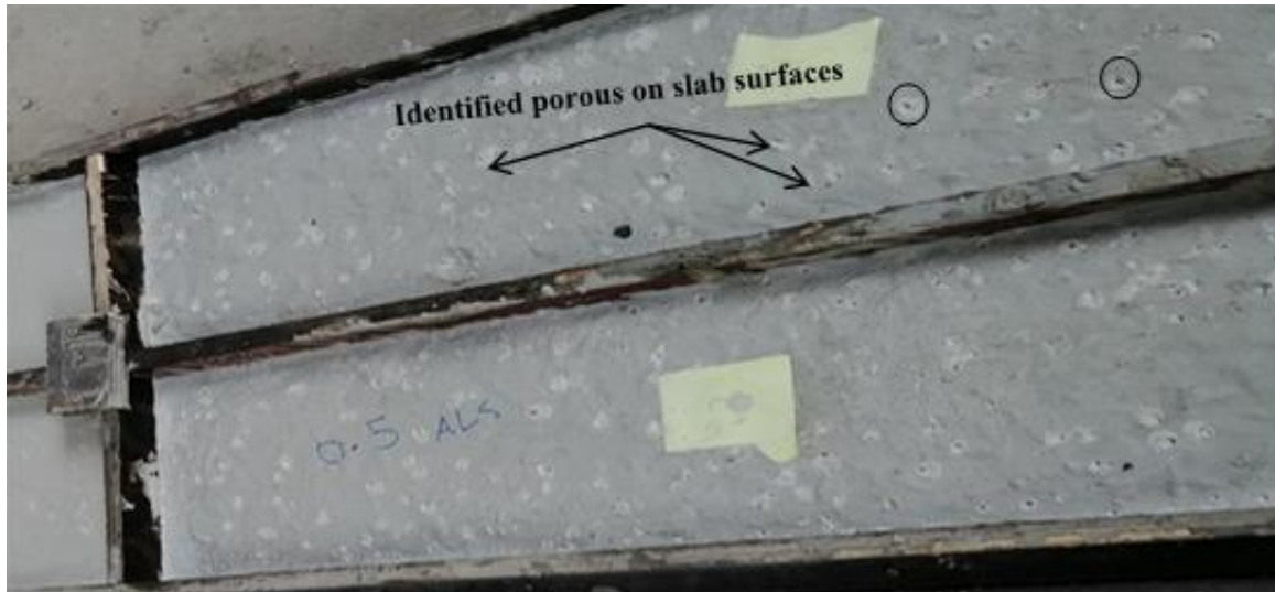
Figure 8. Identified porous on slab surfaces for specimens incorporating aluminum fibers
