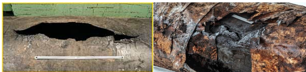
Figure 1. Corrosion in pipes due to high viscosity liquid flow
